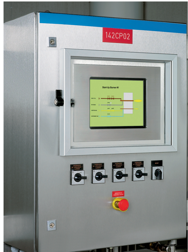
BMS with touch panel for four burners.
